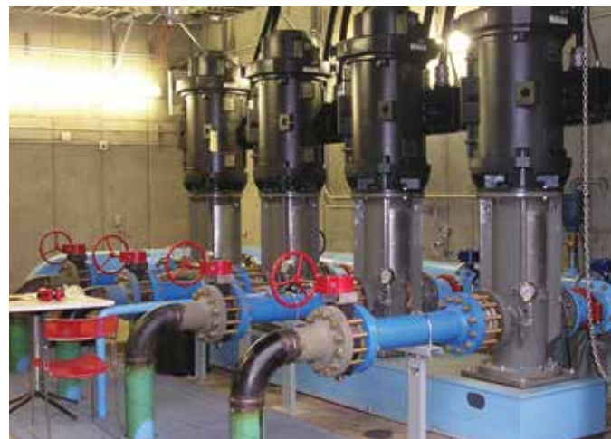
Efficient pumps controlled by variable frequency drives at Highland’s 5 Trees Pumphouse, a project funded by the efficiency fund.
